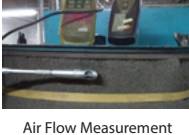
Inlet Air Conditions Measurement
