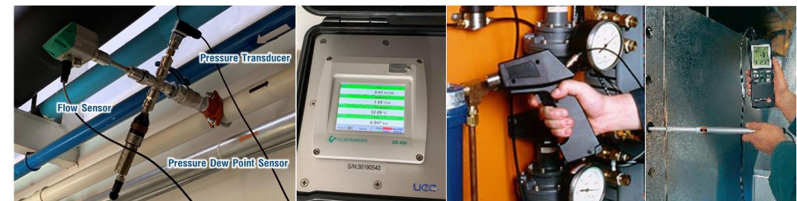
Compressed Air Flowmeters + Pressure Sensor + Pressure Dew Point Sensor with Data Loggers for Dry Compressed Air
